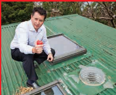
VELUX inspects a roof hit by hailstones the size of cricket balls in the Melbourne storm 2010. All VELUX skylights remained intact.
